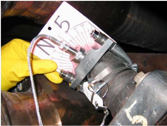
FOLTM Probe on P1 West Reactor Face
